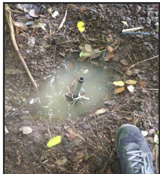
Fig. 29. Water pipes for irrigation
